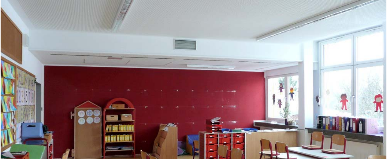
Installation in a ceiling paneling
